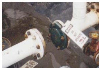
Pipe Blinding Flange
