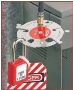
Locked Comp. Air Line
